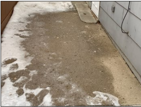
2" concrete repair step at side door.
