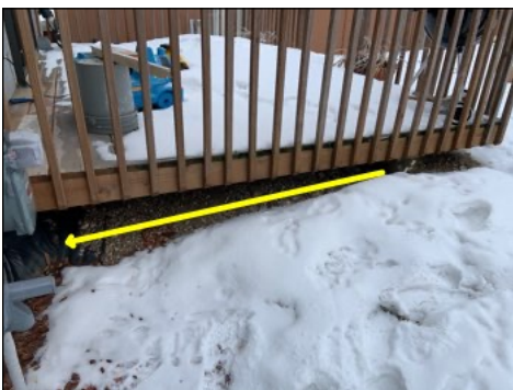
Landscaping under deck slopes toward home. Recommend creating swale in front of deck to divert water away from home.
