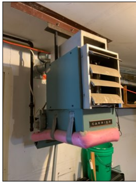
Garage heater not in service.
