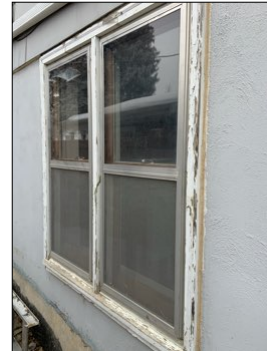
Recommend sealing and repainting trim around windows and doors.
