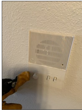
Intercom not operational.
