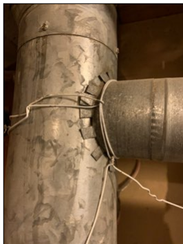
Improper slope and connection on water heater to boiler vent. Recommend repair.
