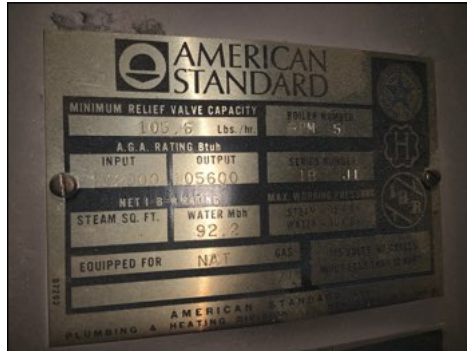
Appears to be original boiler.
