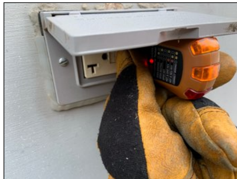
Exterior front does not trip.
