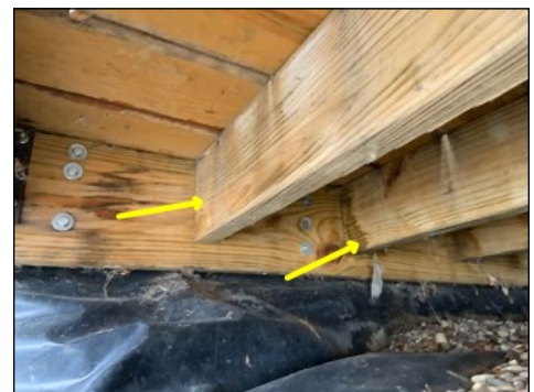
Recommend joist hangers be installed on ledger board.
