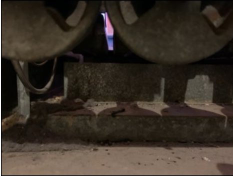
Corrosion in burn chamber. Recommend evaluation.
