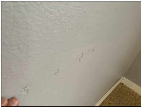
Slight wall damage upstairs
