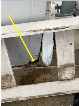
Masonite siding damaged on north side of garage. Recommend repair.
