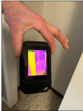
Closet downstairs has signs of past water issue, no elevated moisture nor visible microbial growth.
