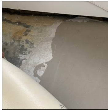
Floor leveler under carpet in downstairs living room.
