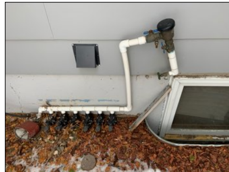
Manifold at rear of home. Recommend covering.
