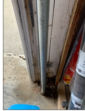
Missing safety sensors.
