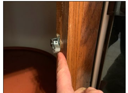
Latch not working upstairs kitchen corner cabinet.
