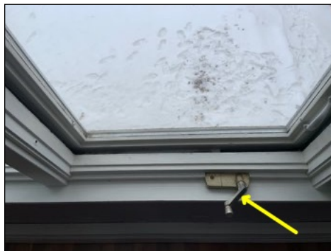
Some loose hardware.
