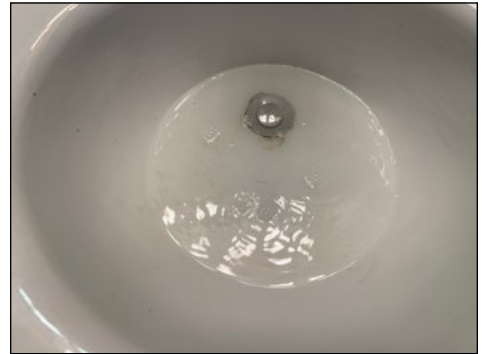
Slow drain upstairs main bat.
