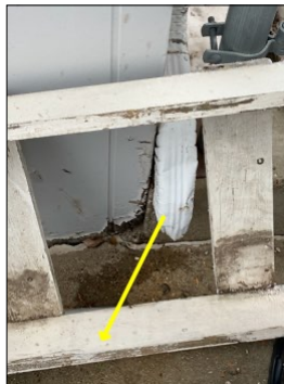
Recommend installing elbow and extension on NE corner of garage.
