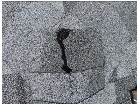
Recommend monitoring and seal all exposed nails.
