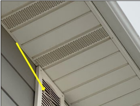
Damaged shutter on front of home. Will be removed when new siding is installed.
