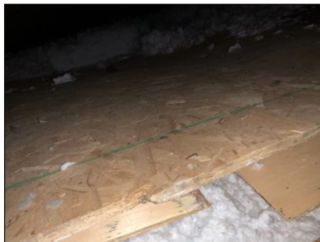
Recommend adding insulation to scuttle hatch.
