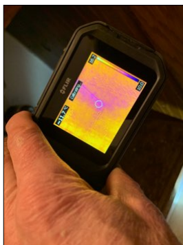
No elevated moisture under downstairs bathroom sink, or along bedroom foundation walls.
