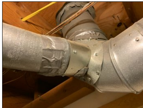
Improper seal. Recommend repair by HVAC specialist.
