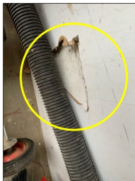
Recommend repair to penetrations in firewall.
