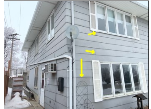
Discolored siding, unsealed joints. New siding will repair areas like this.
