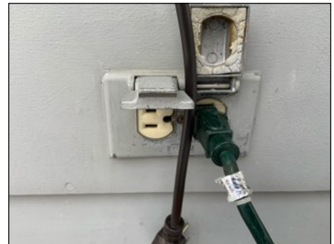
No GFCI in upstairs kitchen, baths, exterior and garage.
