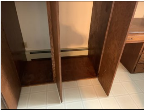
Note heat register behind cabinets in upstairs laundry. Poor heat distribution.
