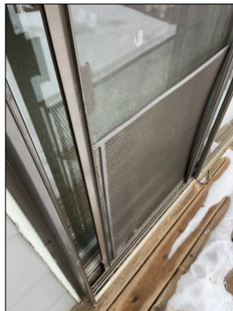
Rear screen door off track.
