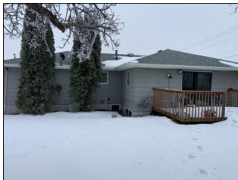
Rear of home includes a deck and main utility entrance. Recommend resloping landscaping to flow away from foundation.
